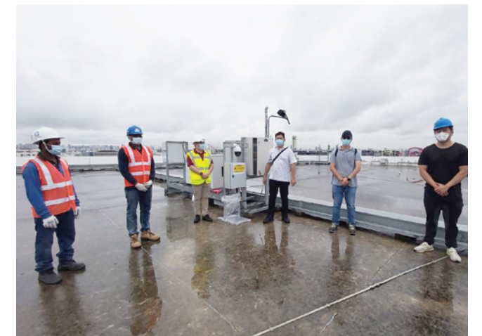
WSH team and contractors installed new remote monitoring system on a rooftop which houses our 5G equipment
